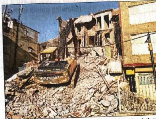
'REFORM NEEDED': Delhi High Court said the property, a stone's throw away from local police booth, had turned from a graveyard to a single-room godown to a two-storey building and then a five-storey building
